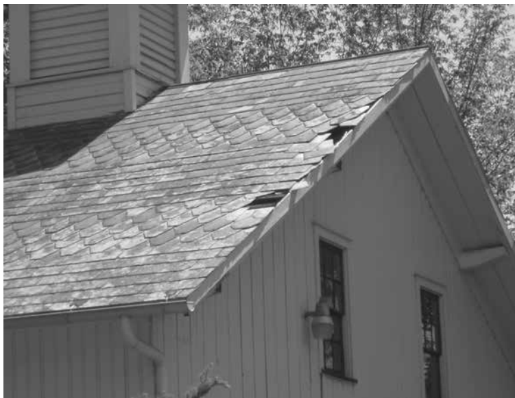
Barn roof holes before the repair work.
